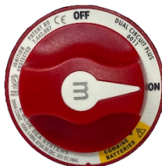
Battery Isolator Switch 'ON'
