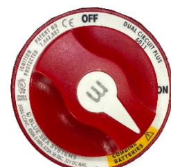
Switch 'Combine Batteries'
